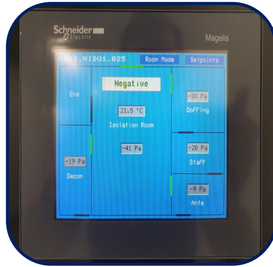
Dual HEPA filtered, sequential negative pressure air handling
