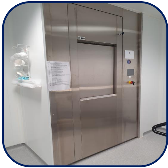
Autoclaves and Cat A Waste Removal
